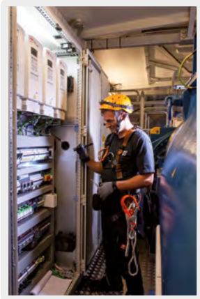
The technician takes a look at the switch cabinet in the nacelle.
