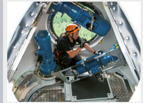
Each rotor blade has its own pitch control system, which aligns the rotor blades individually and serves as a brake and emergency shutdown system.
