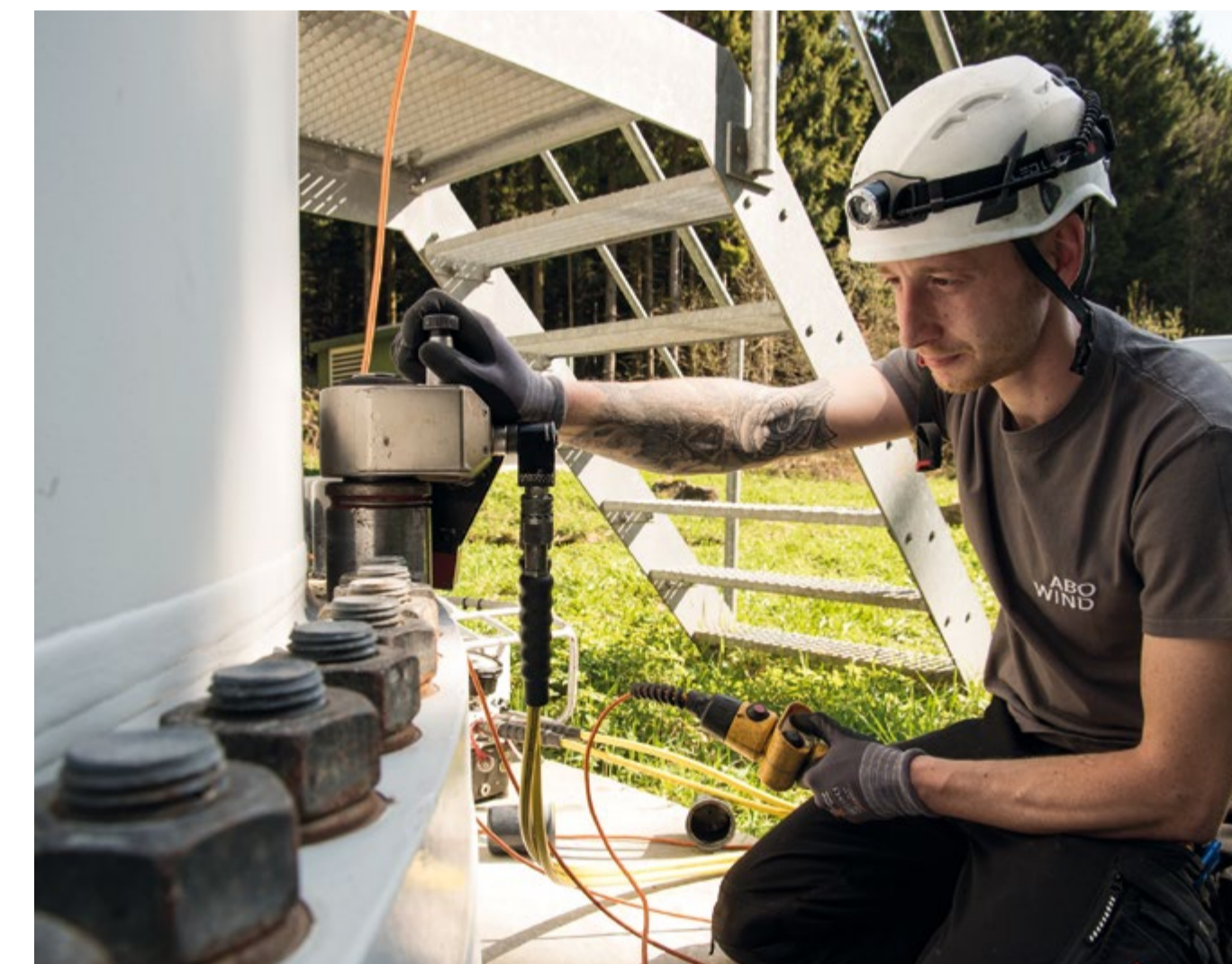
A wind turbine requires safety tests, electrical checks and other maintenance
