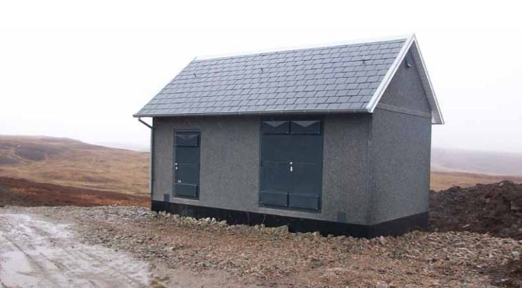
Control Building for Lairg
